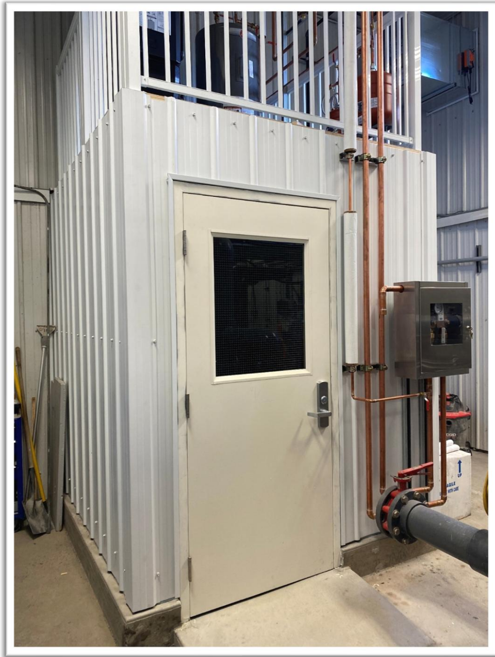
Figure 11: New Chlorine Room
