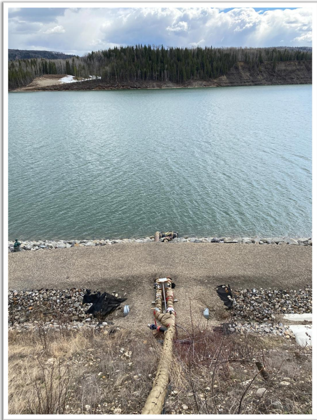
Figure 17: Raw Intake Pipes
