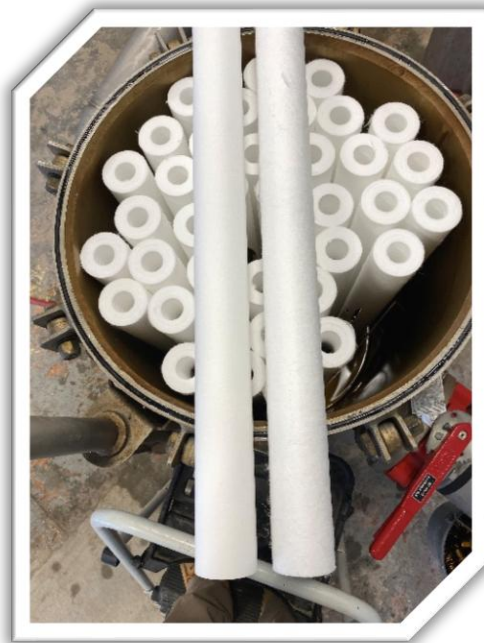
Figure 6: Cartridge Filter Changeover
