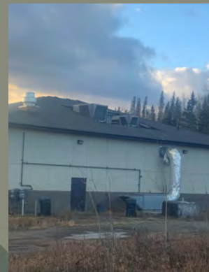
COMMERCIAL FOOD ESTABLISHMENT- ROOF TOP EQUIPMENT
